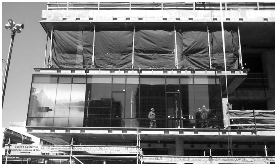
Construction crews install windows on the campus' main building. The window's artwork will feature Chinese images – a visual tribute that speaks to the history and culture of Chinatown.
